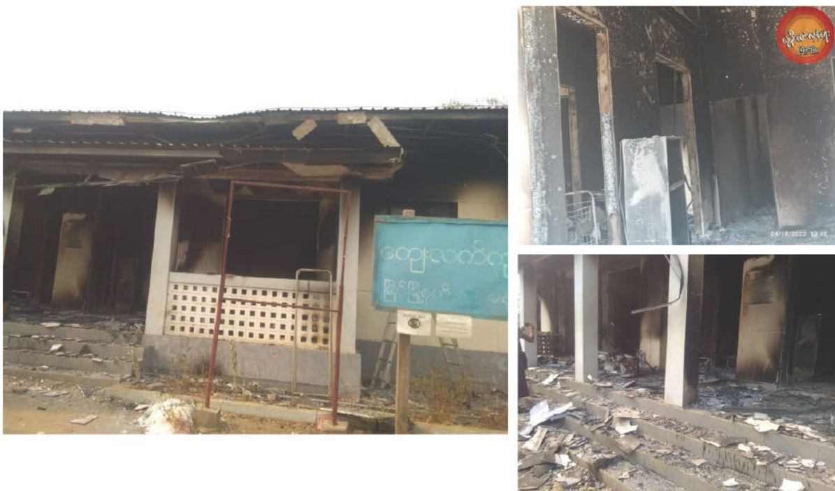
Figure 19: Damage shown from the exterior and interior of the facility shows that the vegetation outside has not been burnt and more fire damage is shown internally and not on the outside walls, suggesting the fire most likely was set from inside (source: Myanmar Labour News ).
