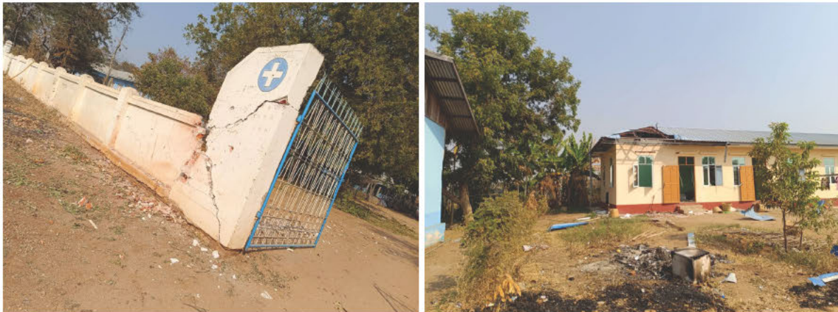
Figure 11: Imagery from the claimed airstrike on Ma Le Thar. (Left) Damage to Ma Le Thar District Hospital wall [22.113461, 95.452112]. (Right) Damage to a nearby medical facility building [22.114029, 95.451988] connected to the hospital (source: Ayadaw Post ).
