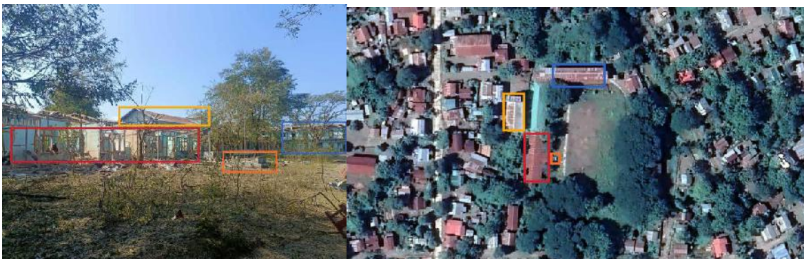
Figure 3: Basic Education High School Ka Nan at 23.805603, 94.144311 was damaged in the attack (Source: Khit Thit Media ).
